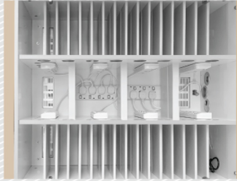
AC power compartment
