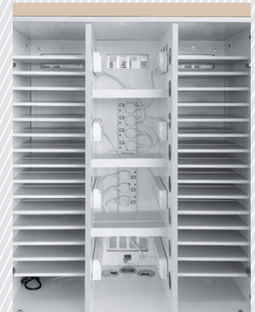
AC power compartment
